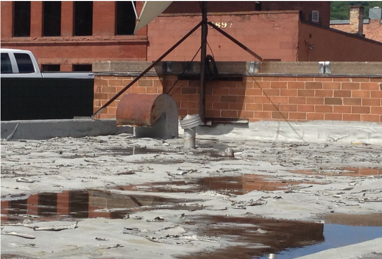
Efforts to raise money for a new roof are ongoing.
